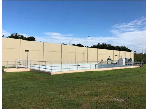
CHLORINE CONTACT CHAMBER
