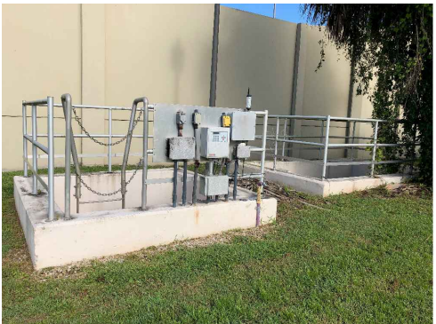
FLOW METER VAULT AND OVER FLOW STRUCTURE
