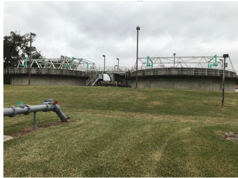
PRIMARY CLARIFIERS NO. 1 (LEFT) & NO. 2 (RIGHT)
